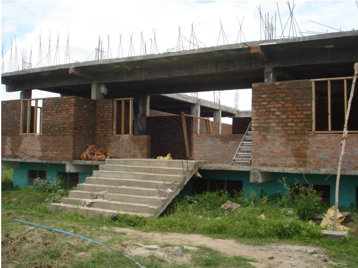
The outer walls of the parish centre being built in brick (hospital underneath)
